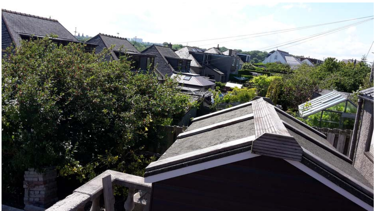
View of the rear of properties at Donmouth Road from Donmouth Crescent showing all rear dormers line up.
