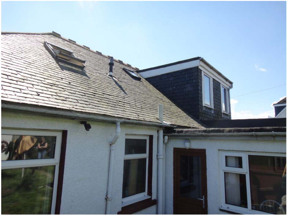
Looking towards rear side of No 5 Donmouth Road. It is planned that the proposed rear dormer will line up with the existing neighbouring dormer
